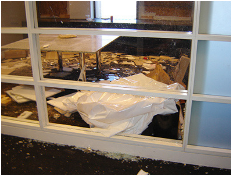
Damage to approximately half of 100 Peachtree's 44 tenants' spaces included fallen ceiling tiles, knocked-out interior walls, and broken windows. Floor plans
